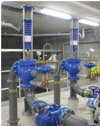
REGION OF PEEL INSTALLATION - ONTARIO, CANADA
