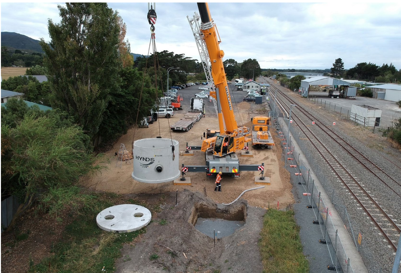
FIG. 5 18 module Up-Flo inside a 3.0m dia manhole treating a 6,500m 2 carpark at Featherston Railway station. Credit SDCL for image.
