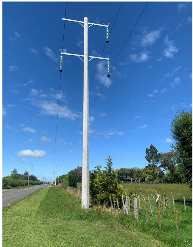
FIG. 3 | Octagonal power pole
